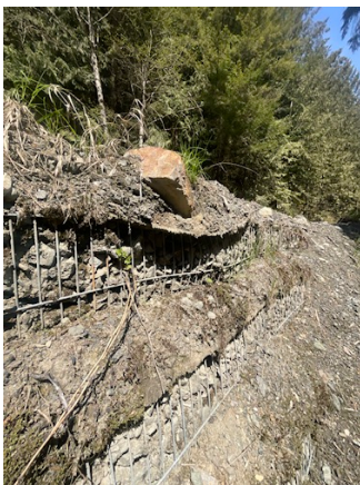
Some bulging upper 2
